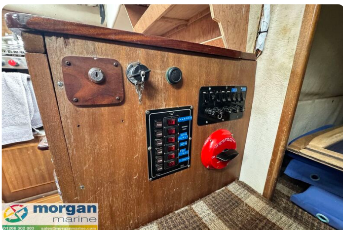
Westerly Griffon MK1 - switch panel
