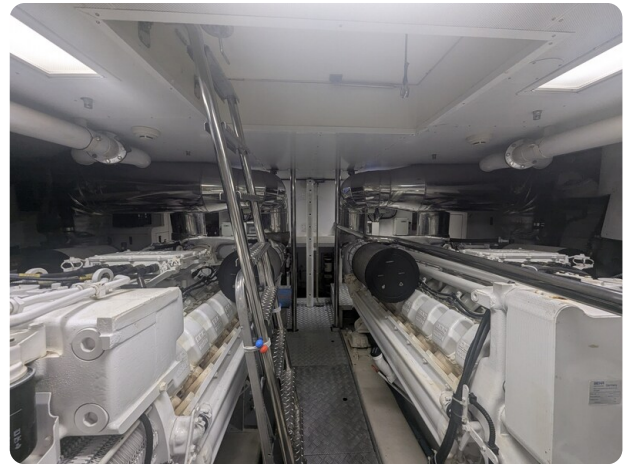
Riva 85 Opera engine room
