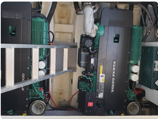
Beneteau MC5 engine room
